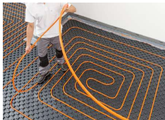
Hot water under-floor heating
